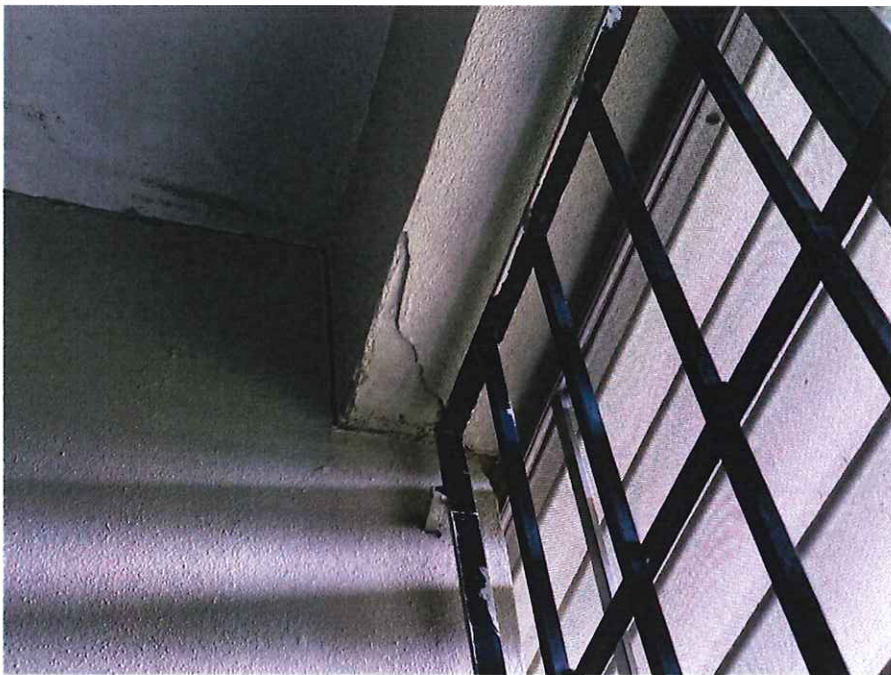
Photo 2: Crack at ceiling/column intersection
