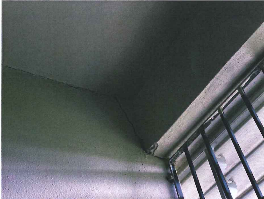
Photo 3: Crack at ceiling/column intersection
